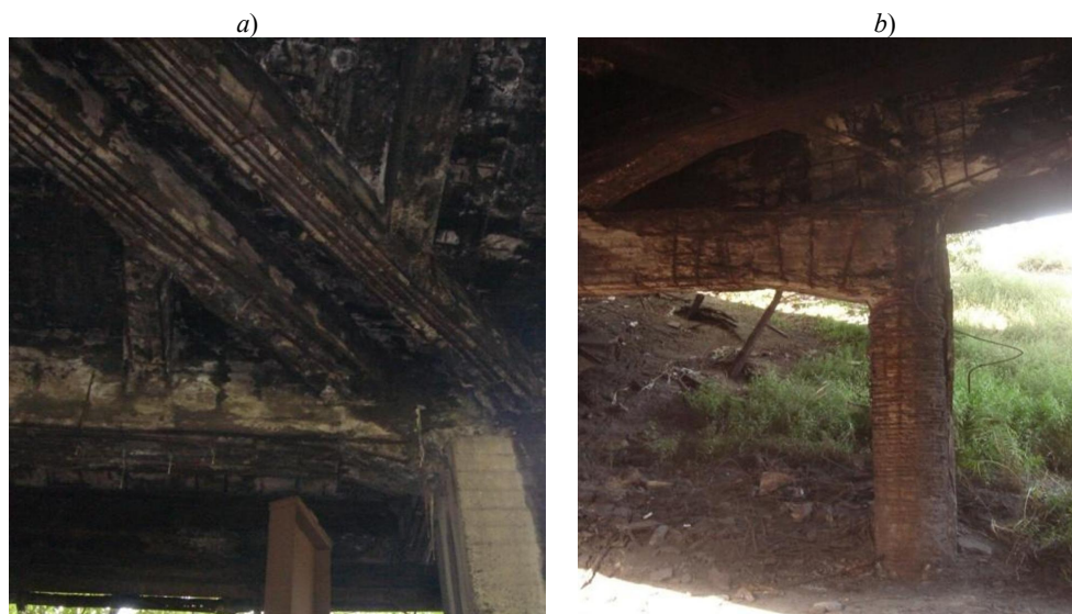
Fig. 1. Damage of reinforced concrete girders (a, b) and supports (b) of the pipeline within the territory of PJSC MMK Azovstal (Mariupol) in the area with high content of sulphur dioxide and carbon dioxide in the air.
